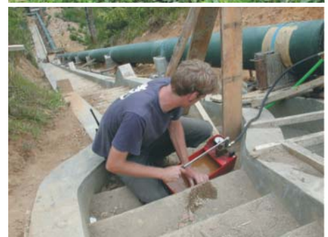
Pressure testing of the penstock pipe. The net head of the scheme is 62m and the penstock has a total length of 194m.
