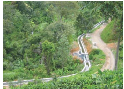
The 572m long stone masonry headrace channel connects the intake with the storage tank. It runs alongside the estate road and features a number of aqueducts and pipe bridges.
